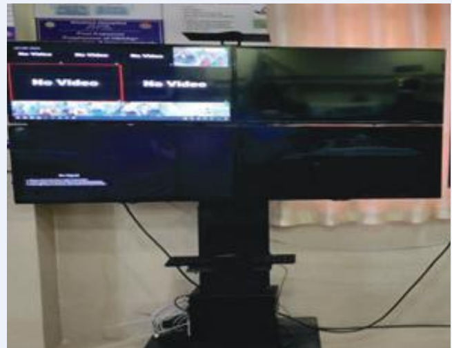
Hardware Installed at Spokes
