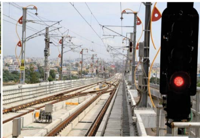
Metro Rail technology –signalling and communication system
